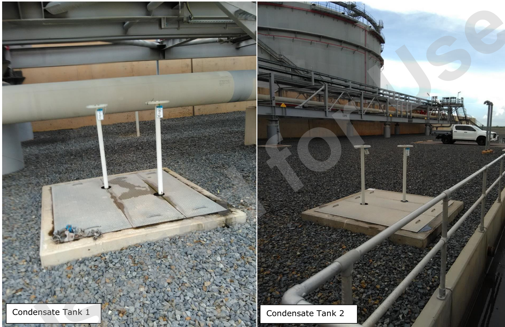
Figure 4-1: Condensate tanks bund drain isolation valves
