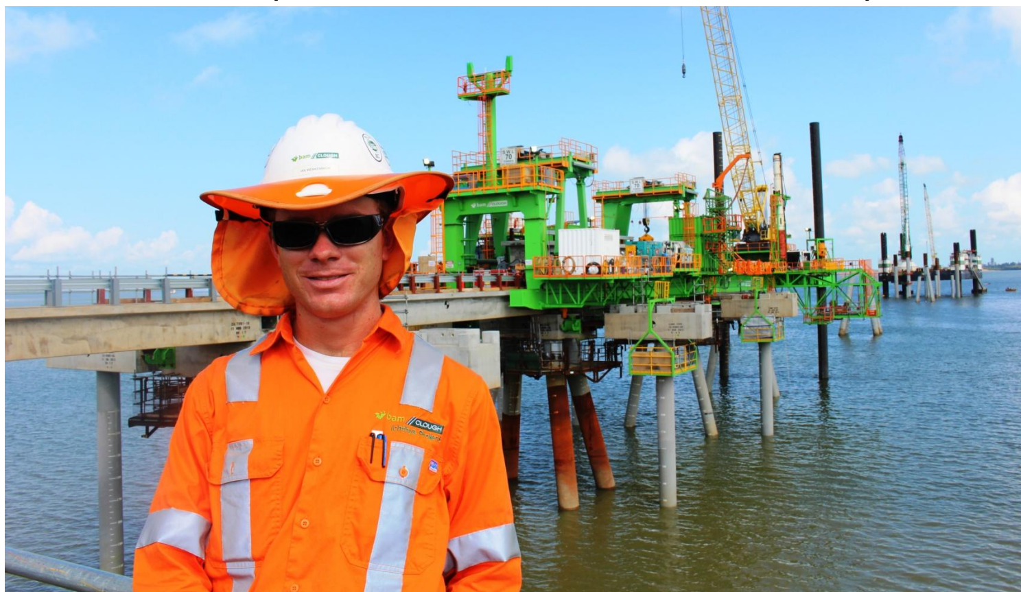
BAM Clough's Ian Wenkenbach in front of the cantilever bridge which is being used to construct the jetty.
