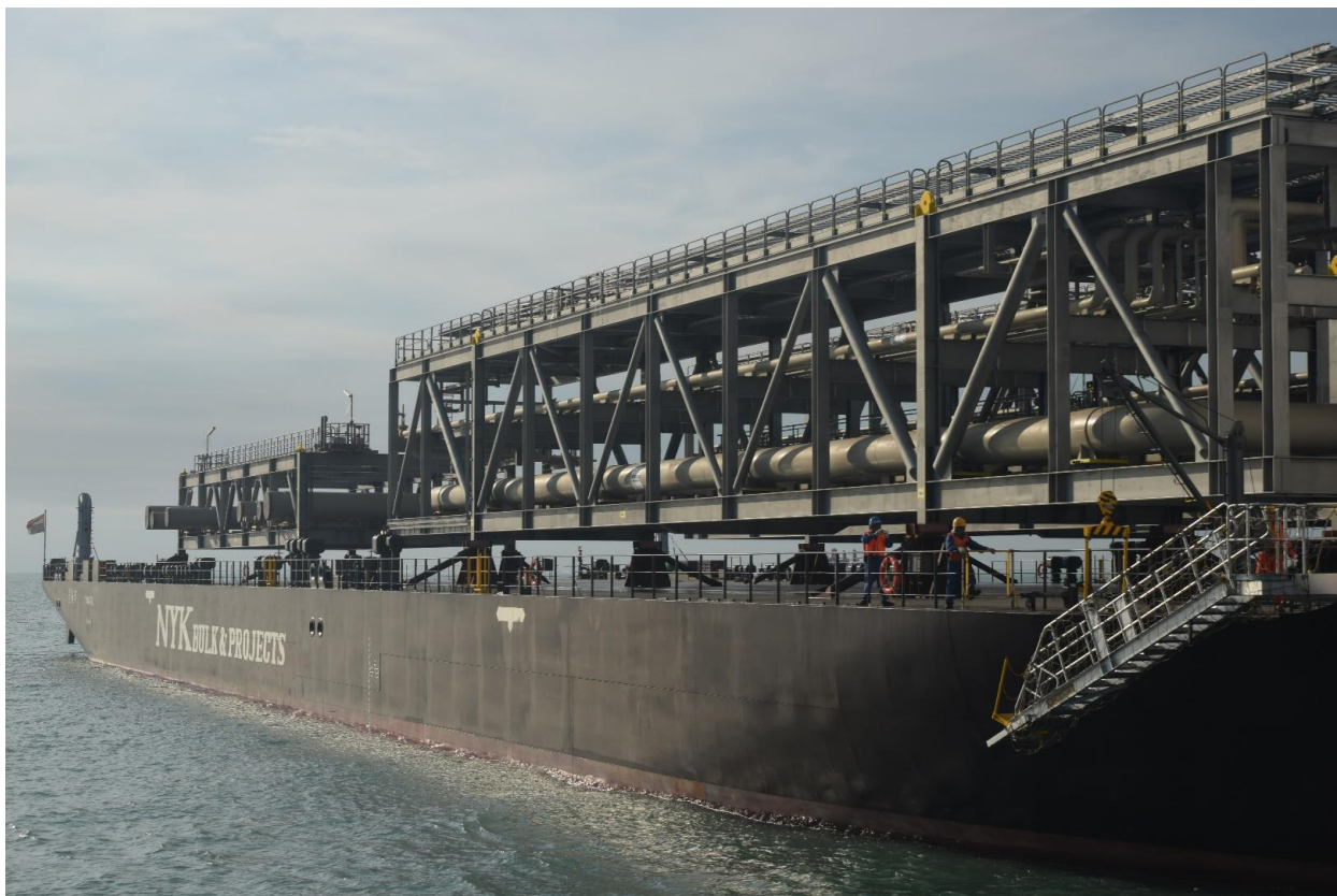
Above: the first of more than 200 very large modules will arrive at the module offloading facility (MOF) next week.
