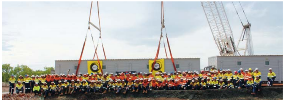
Project workers at Manigurr-ma Village celebrate the safe installation of the last over-sized module
